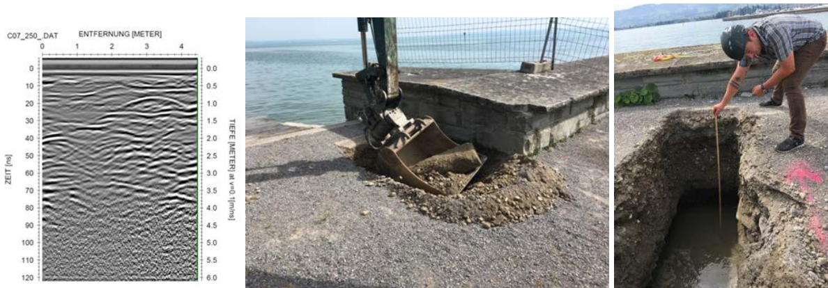
Fig. 12): The Profile C7 has a distinct hyperbola (picture left). The excavation brings out a large stone block (middle picture). The remaining excavated material consists of round stones of 3 - 5 cm diameter with little finely granulated material. The water flows immediately (picture right).
