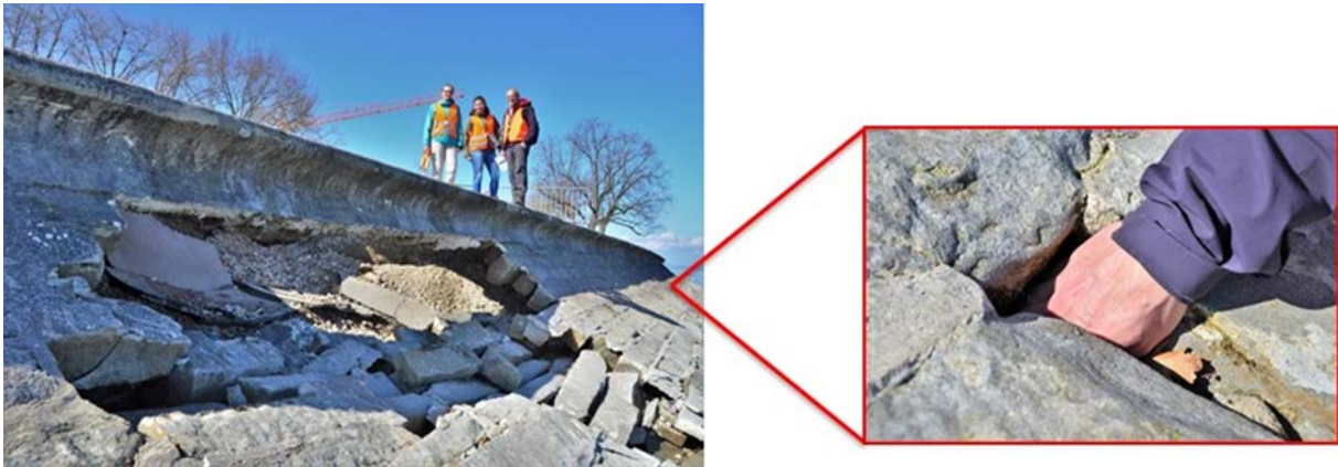
Fig. 4): Collapsed site near the promenade (left). Holes between the stones in the ramp (right).
