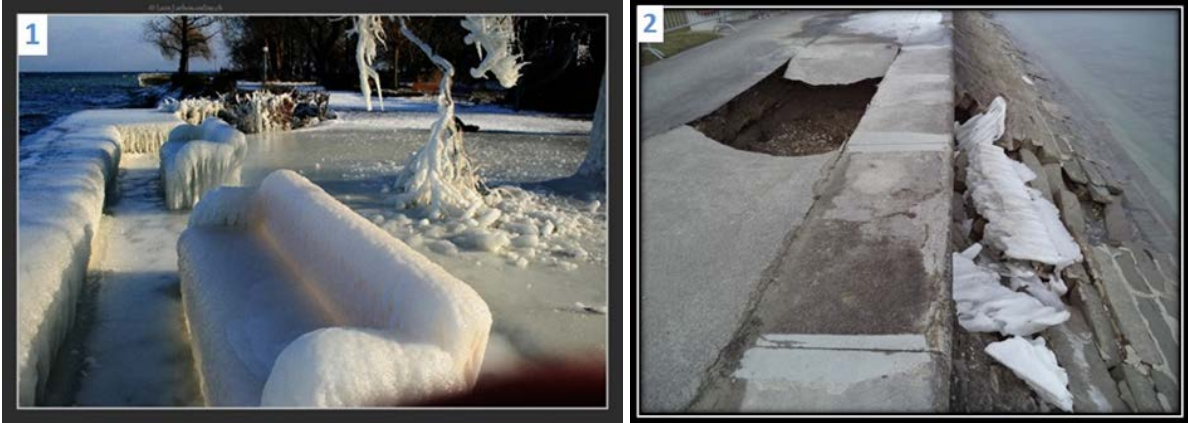
Fig. 3): Ice shield on the shore in February (left) [4]. Collapsed ground after the melting of the ice in March 2018 (right).
