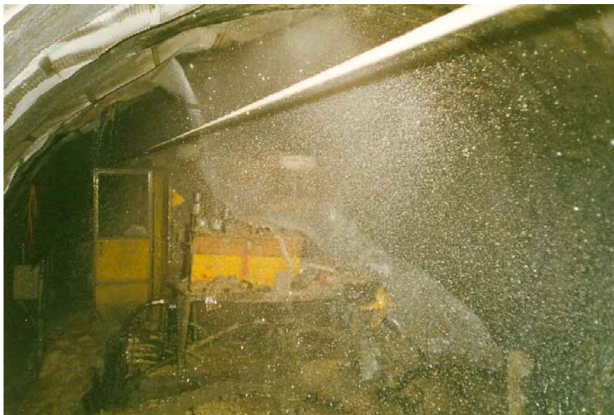
Fig. 10: Blow-out from borehole at 5553 m. A mixture of sugar grained dolomite and water with 1000 m overpressure filled the tunnel. Photo R.Volpers [6]
