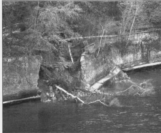
The broken quay wall, a short time after the slide occurred. It was not clear whether the breach of the wall was a consequence of the slide or vice versa. This event happened during the day without any precursor.
